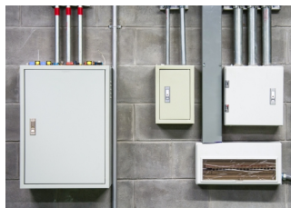
Branch Distribution Panels
