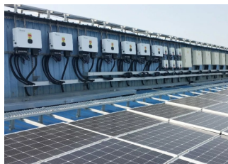
Inverter DC Input Side
