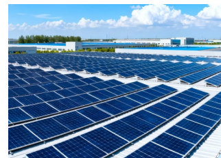
Commercial Rooftop PV Systems
