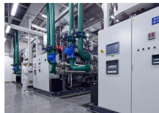
Industrial Control Systems
