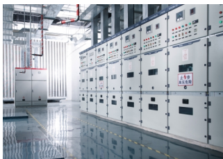
Building Main Distribution
