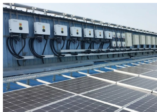
Inverter DC Input Side
