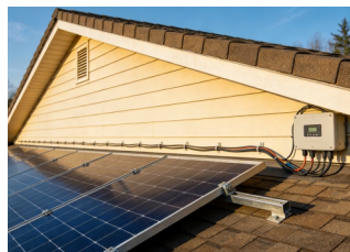
Residential Rooftop PV Systems
