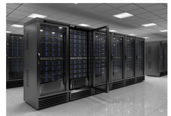
Telecom & Data Rooms
